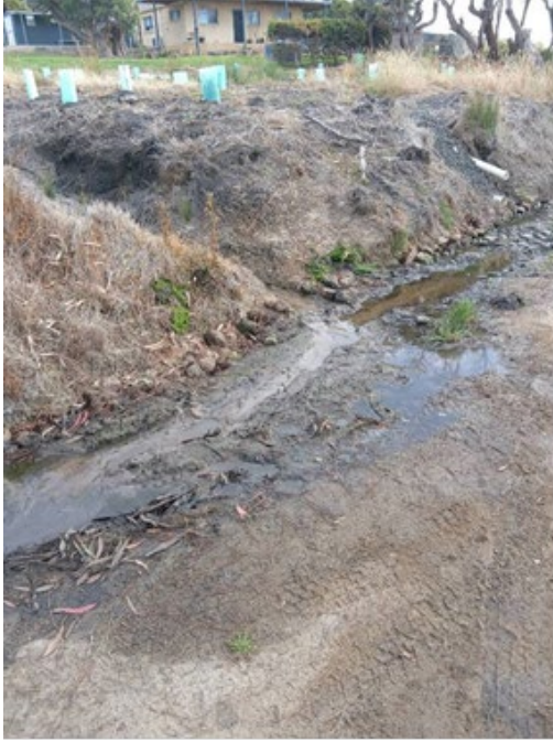
Seepage running onto Primrose Beach near the boat ramp
