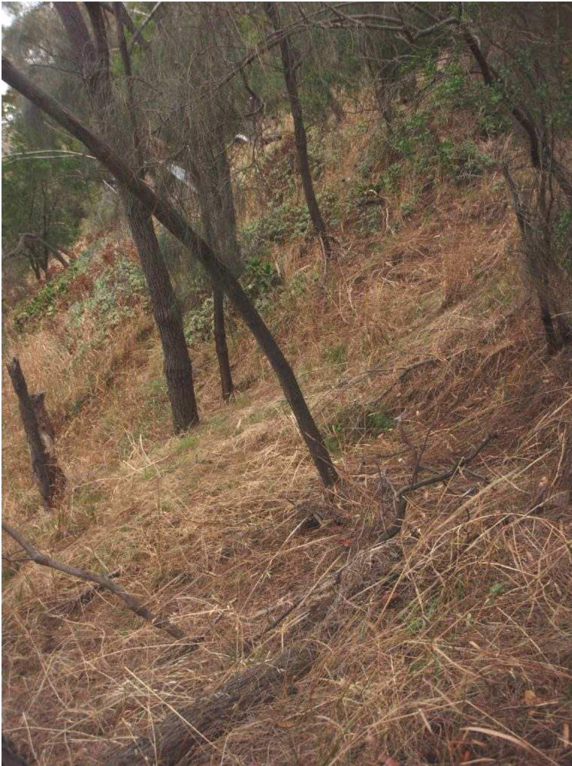
Plate 3 (above). View southwest across the 30 – 35° slopes of the embankment below 513 Shark Point Road. Hummocky ground and leaning and curved tree trunks indicate shallow-seated slope instability (mainly soil creep and small scale landsliding)
