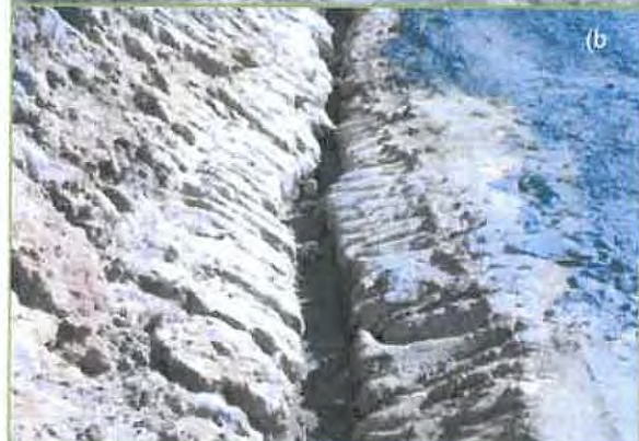
Figure 6 (a). Tunnel erosion resulting from construction of a culvert in dispersive clay (b). Tunnel erosion caused by installation of optical fibre cable in dispersive soil.
