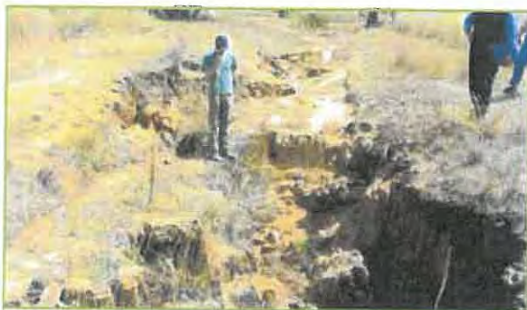
Figure 1. Tunnel and gully erosion resulting from construction of a stormwater culvert in dispersive clay.
