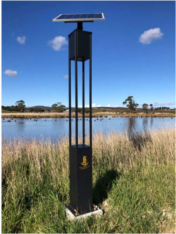
Figure 1 - Solar Powered Down Lights
