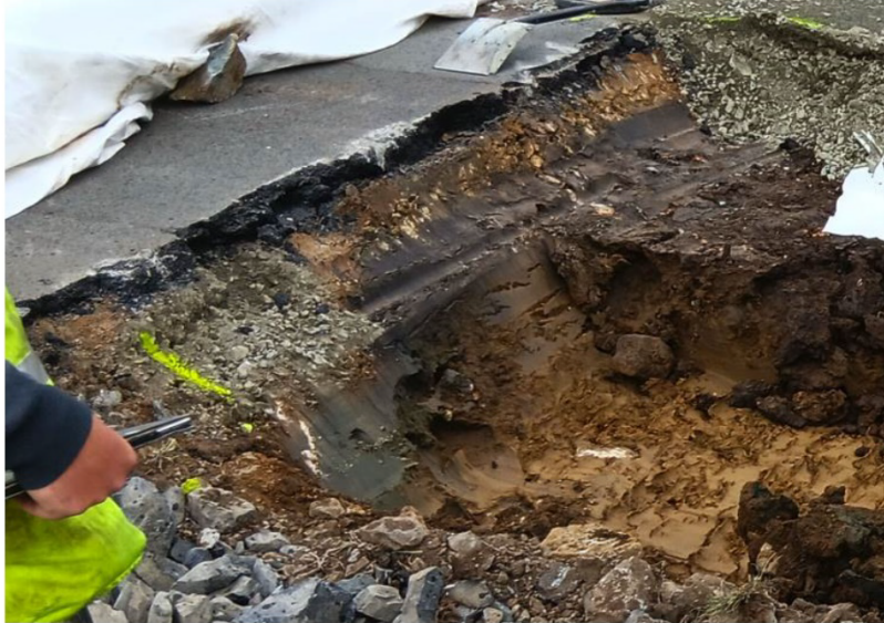
Figure 1: Existing road pavement transition at south extent of works on Primrose Sands Road
